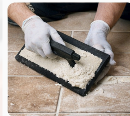
Applying epoxy grout into tile joints using a rubber grout float at a diagonal angle.
